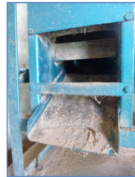
Huller exit port - dusty & not cleaned for many days
