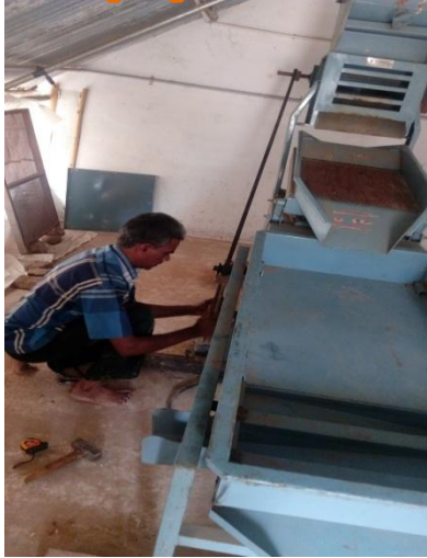
Fitting destoner at Pudur Nadu
