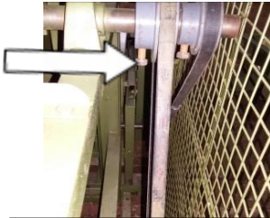
Fig. 17: Avoid use of hex head bolt for securing pulley to the shaft
